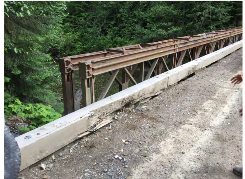
Guard Rail damage noted at down stream left approach
