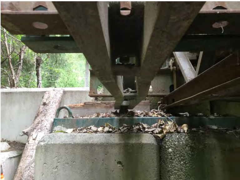
Down stream. Right bank chord condition
