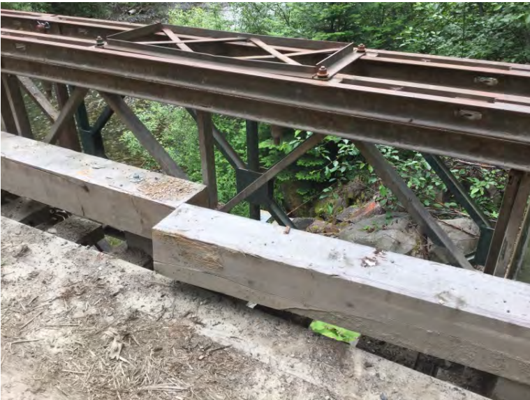
Up stream left approach guard rail missing hardware
