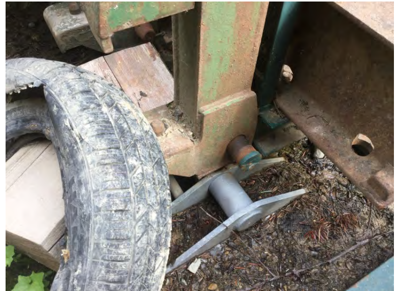
Upstream left approach pin loose
