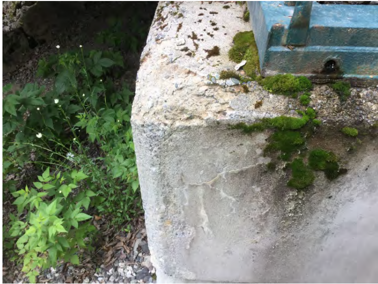
Right upstream lock block spall
