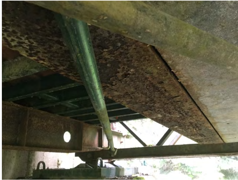
Transom corrosion - typical
